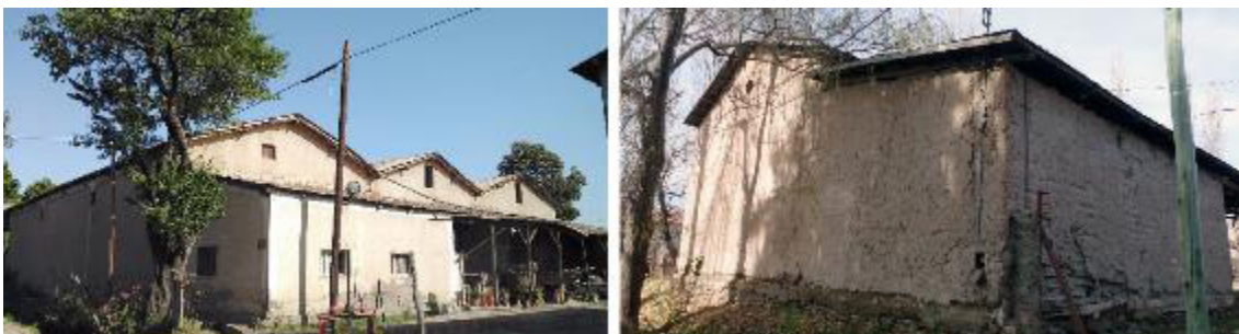
Figura 5. Izquierda: bodegas con revoque cementicio. Derecha: bodega con revoque de barro y paja Figure 5. Left: winery with cementitious plaster. Right: winery with clay and straw plaster
